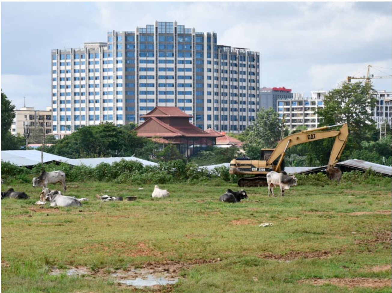
Construction of Shwe Kokko new town in Karen BGF-controlled territory on Thailand border (TNI)
