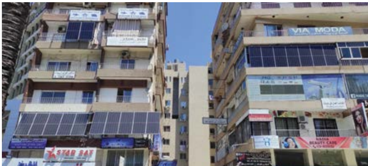
Figure 1: Solar panels on balconies in Beirut (Photo: authors)
